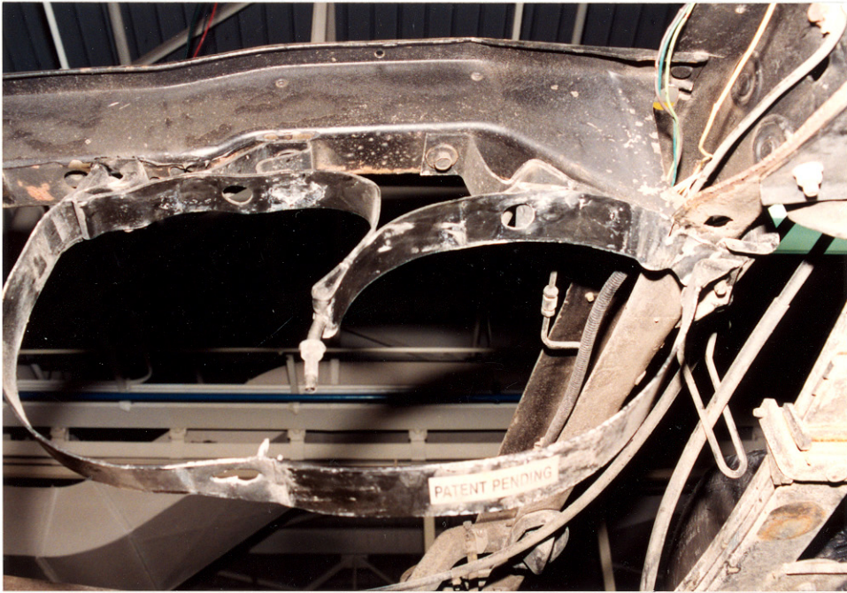
29. View of the combined rear attachment strap for the failed CNG tank (on the right side of the photograph) and the center tank looking rearward
